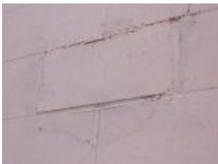
Top: Dislodged block, exterior wall. Below: Cabinet against exterior wall.
