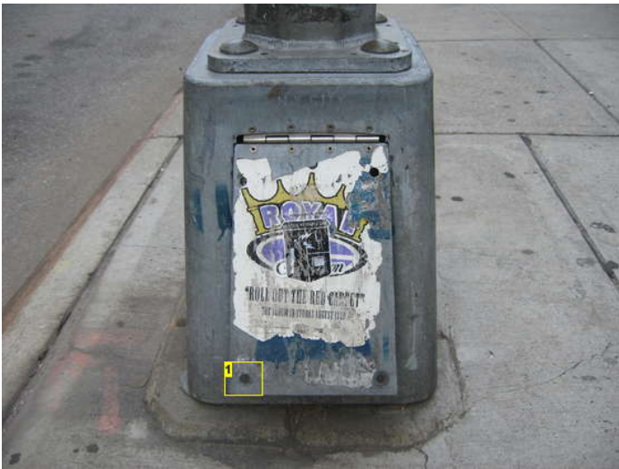
Image Notes 1. look for missing bolts
