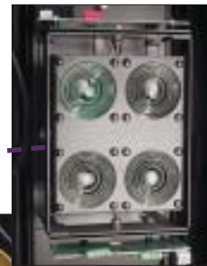
MICROWAVE DEVICE The microwave coverage is provided by a microwave transmitter and a receiver using parabolic antennas. The coverage pattern can reach 490 feet, and 19 feet in diameter.
